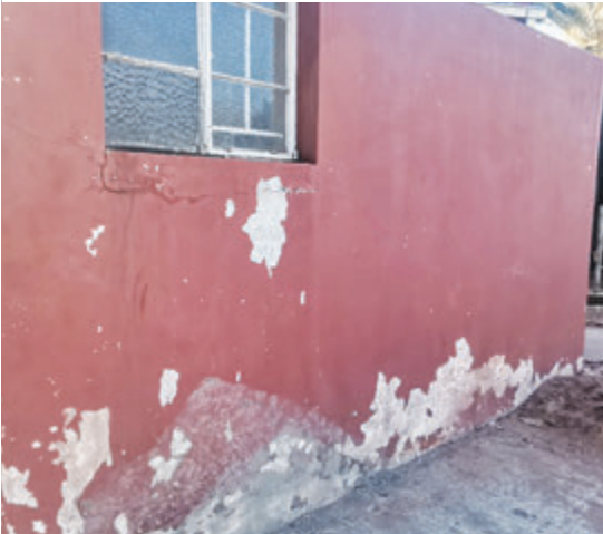
The home needs of a fresh coat of paint.
