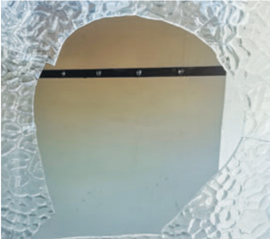
The old, broken windows need to be replaced.
